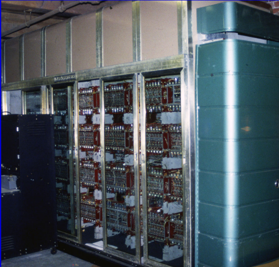
Central Processing Unit
